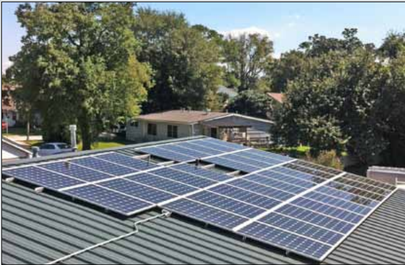
A rooftop solar installation generates clean energy in New Orleans.
